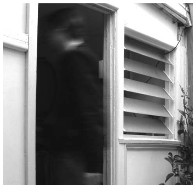
Asbestos cement sheeting used on an exterior wall.
