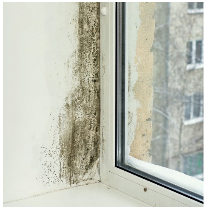
Figure 1 Mould on a wall
